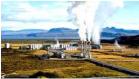
Nesjavellir Geothermal Power Station
