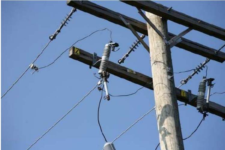
Gambar 2.6 Fuse Cut Out
