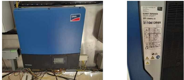
Fig. 3. Inverter Ongrid 17 kw at Lab RE IT PLN
