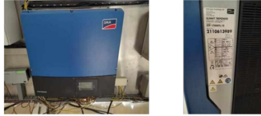
Fig. 3. Inverter Ongrid 17 kw at Lab RE IT PLN
