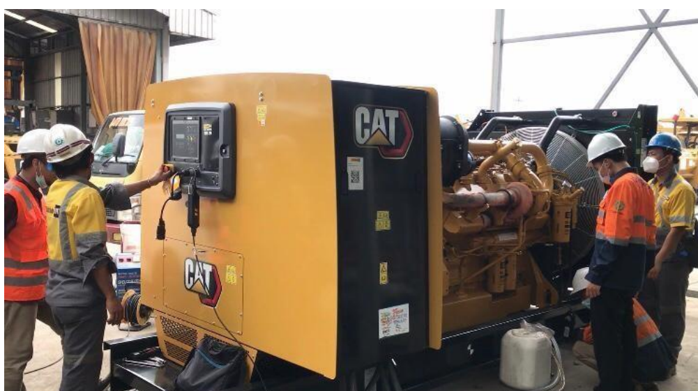
Gambar Starting Genset
